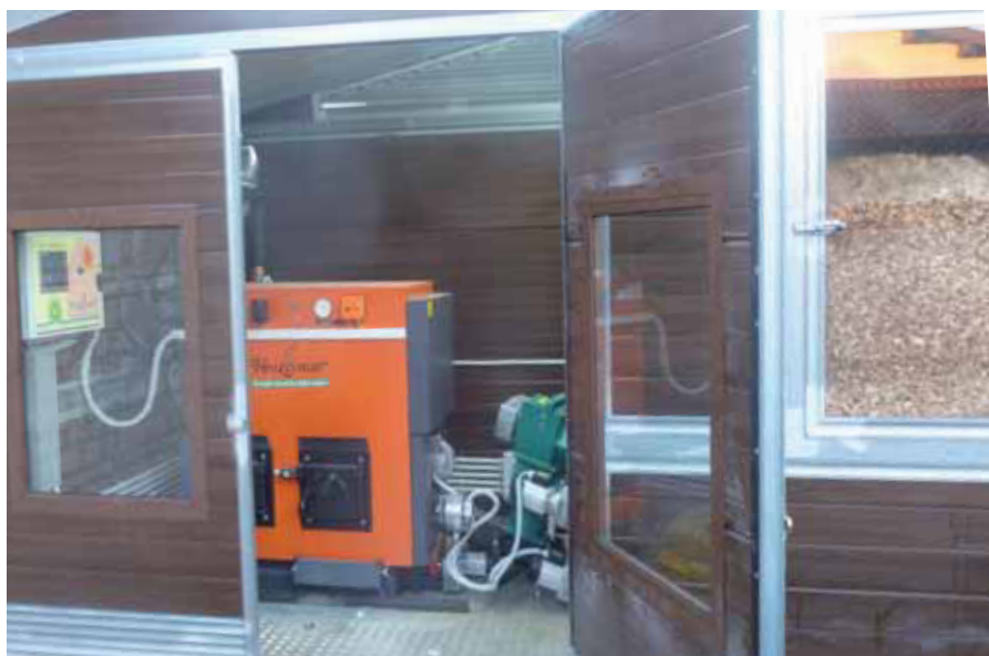
La caldaia in container Heizomat HSK-RA 34
